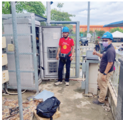
Configuration and Installation of network equipment in Base Transceiver Station
