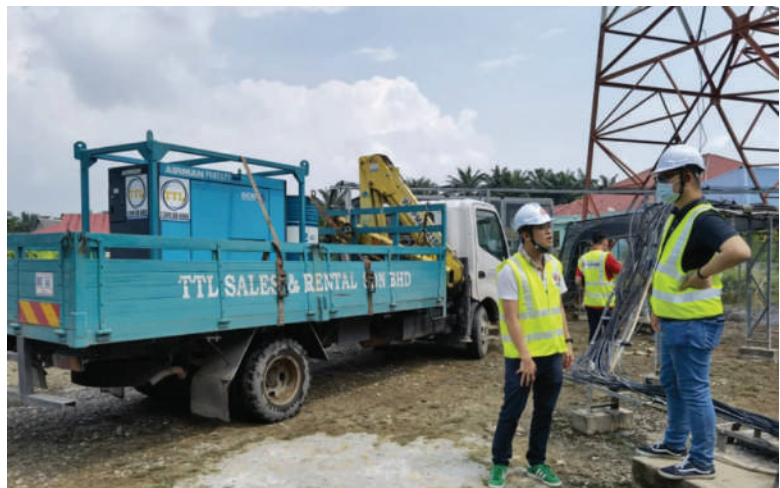
Installation of Mobile Generator Set (Gen Set) at the Affected Communication Structure
