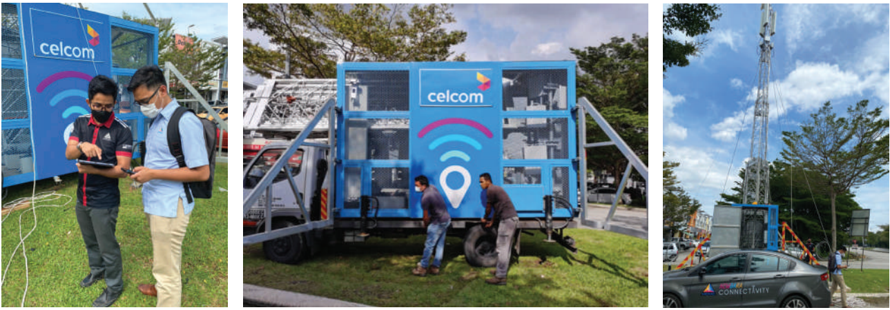
Installation of Coverage on Wheels (COW) - a mobile transmitter system to provide temporary service coverage while MCMC SSO officers perform quality test
