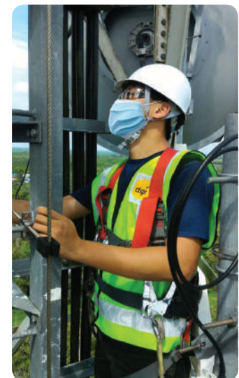
Digi's network team on-site strengthening 4G network
