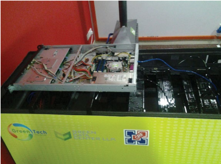
Servers operating with Eco2
